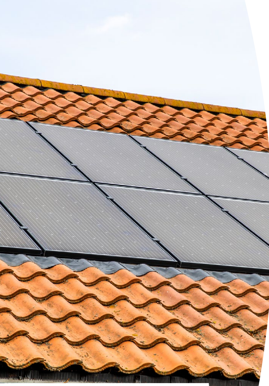
Solar panels at Hadleigh Country Park
