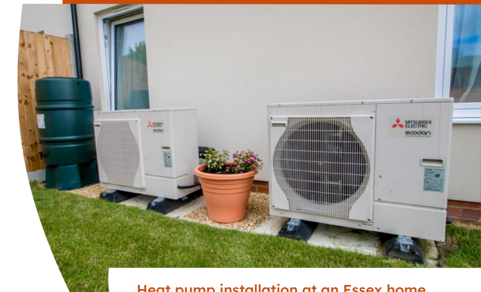
Heat pump installation at an Essex home
